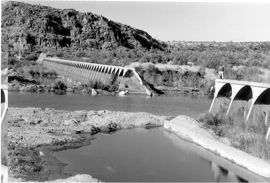
Figure 18.11 Photograph of sediment above and below Gillespie Dam, Gila River, Arizona, with human figures on the dam crest for scale. The sediments behind (to the right) the dam had accumulated to a level slightly above the crest before the breach. WL. Graf photograph 127-22, 8 December 1994
